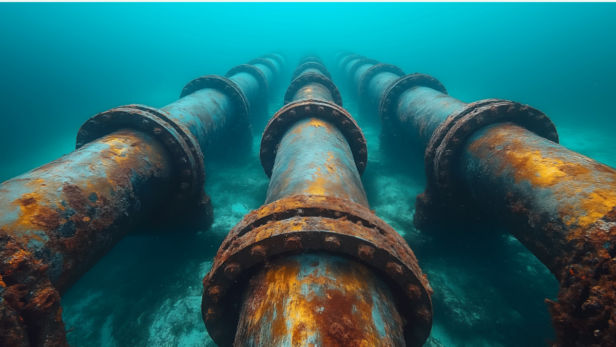
A gas pipeline
